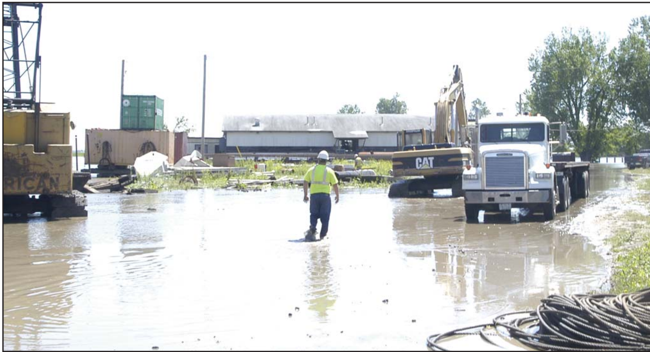
Mike Habegger, manager of the Rulo bridge project, stated that flooding has slowed the progression and as of Tuesday, is at a standstill. The Main Span contractor has been waiting nearly a month to begin work because of heavy rains and Missouri River flooding.
